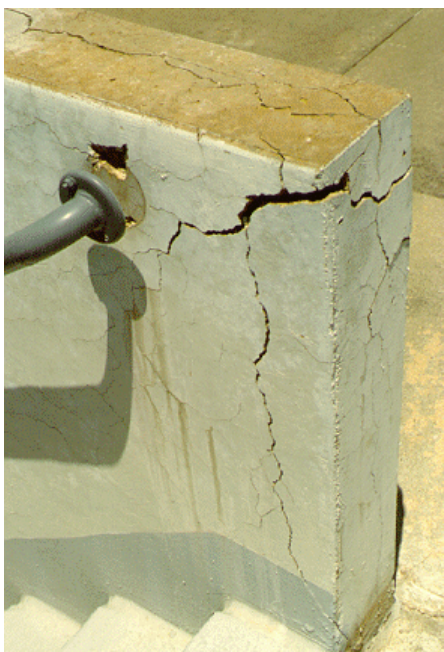
Figure 2.13: Severe concrete cracking attributed to delayed ettringite formation [Myers, 1998]
