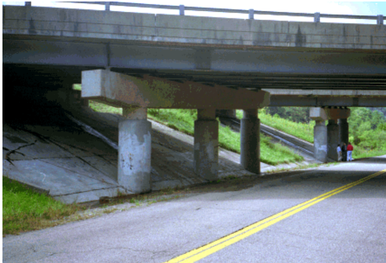
Figure 1.1 A deteriorated bridge pier & deck on Highway 44
