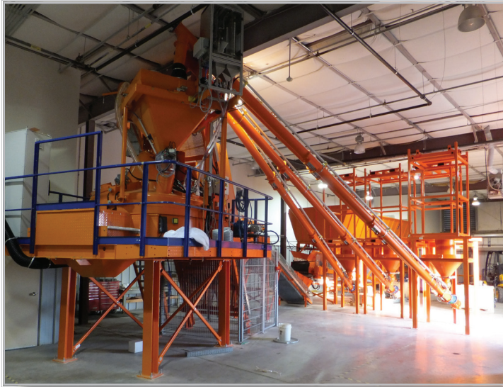
CTIS Concrete Batching Plant
