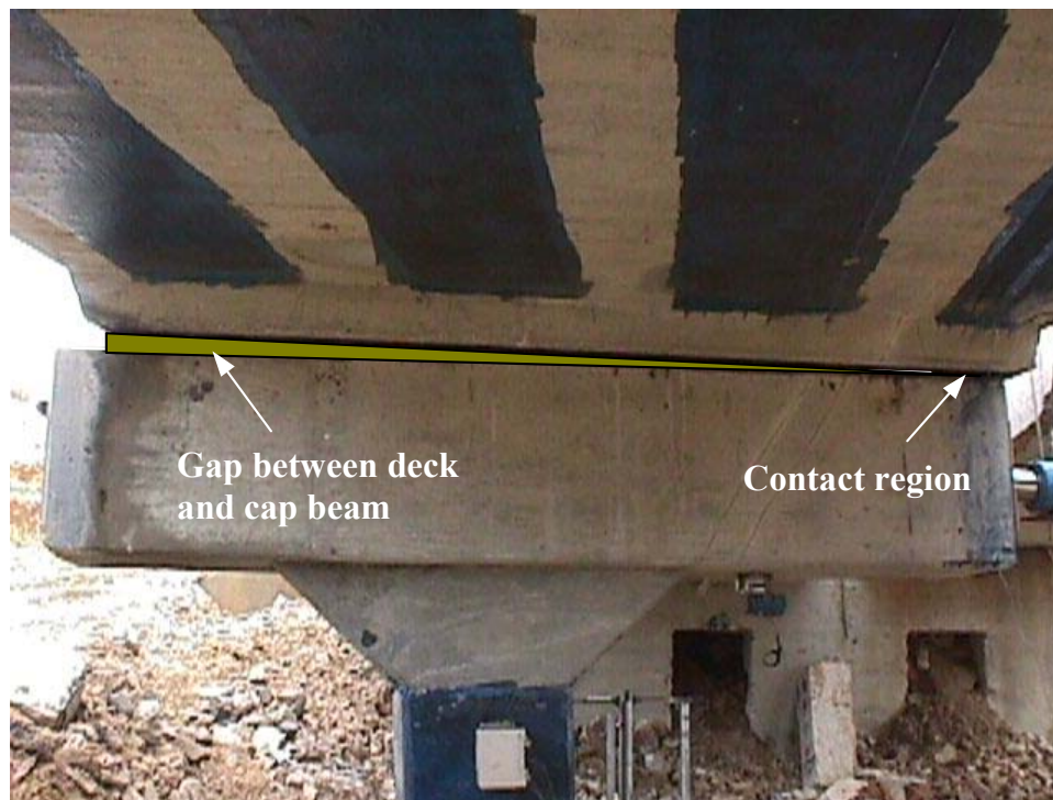
Figure 4.32. Rotation of the cap beam relative to the topping deck.
