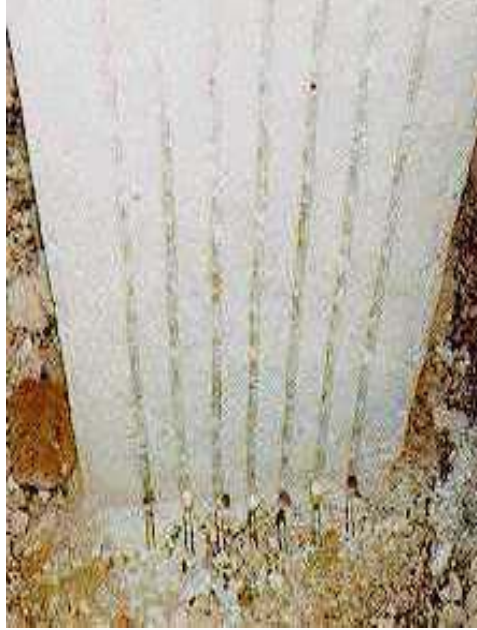
Figure 2.9. Drilled holes at the base of column B2P2 for anchorage of CFRP rods.
