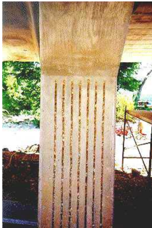
Figure 2.8. Grooves on the side of column B2P2.
