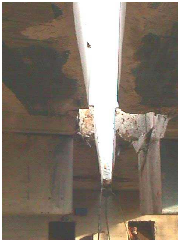
Figure 3.3. The bridge deck and a cap beam after cutting and removing concrete.
