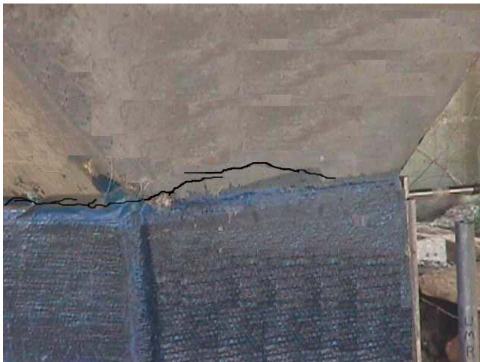
Figure 4.33. Crack at column/haunch intersection at failure.
