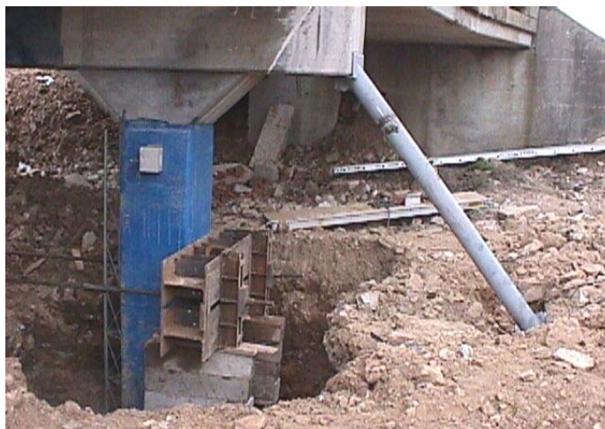
Figure 3.18. Diagonal bracing of the failed column.
