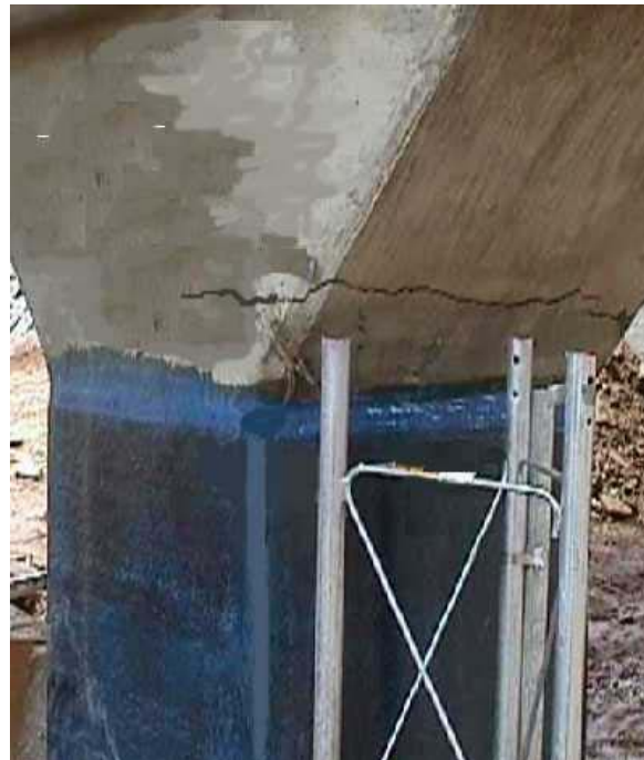
Figure 4.13. Crack at failure of column B2P2.
