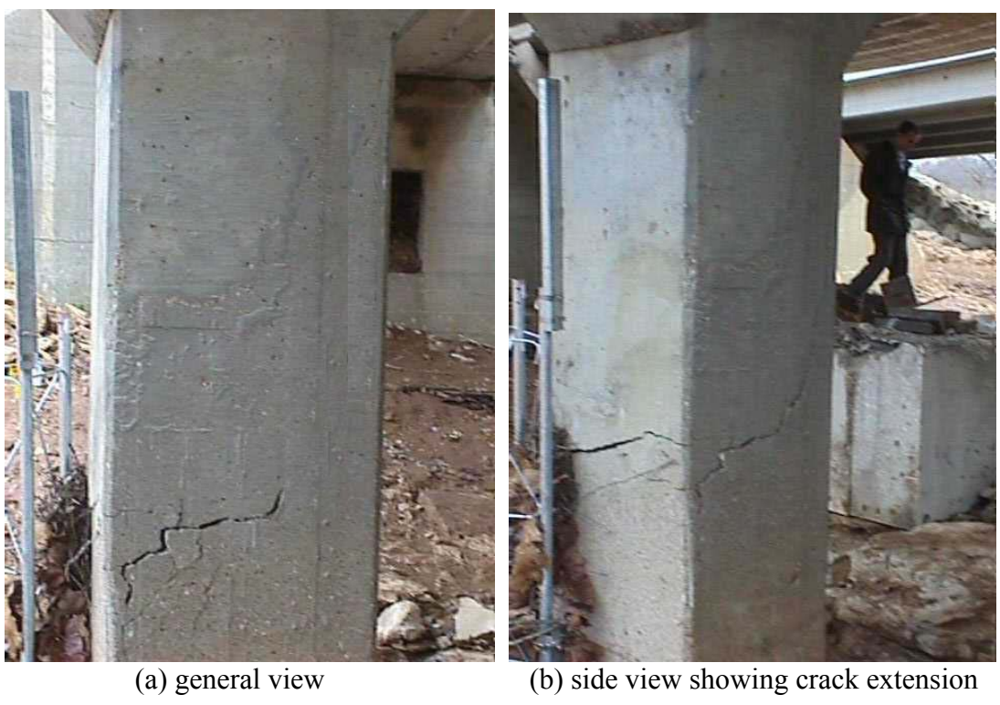
Figure 4.7. Crack on Column B2P1.
