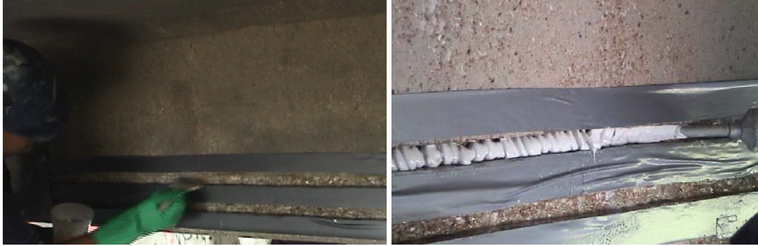
Figure 14. Epoxy resin and epoxy adhesive in slot cut in the concrete surface
