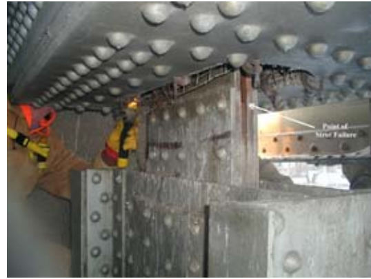
Figure 4 Point of Strut Failure
