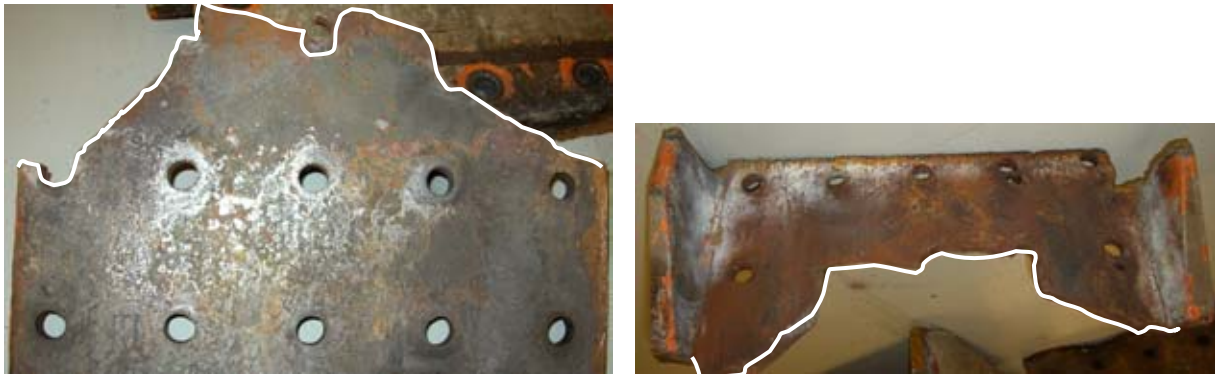
Fig. 11 Line of Strut Fracture
