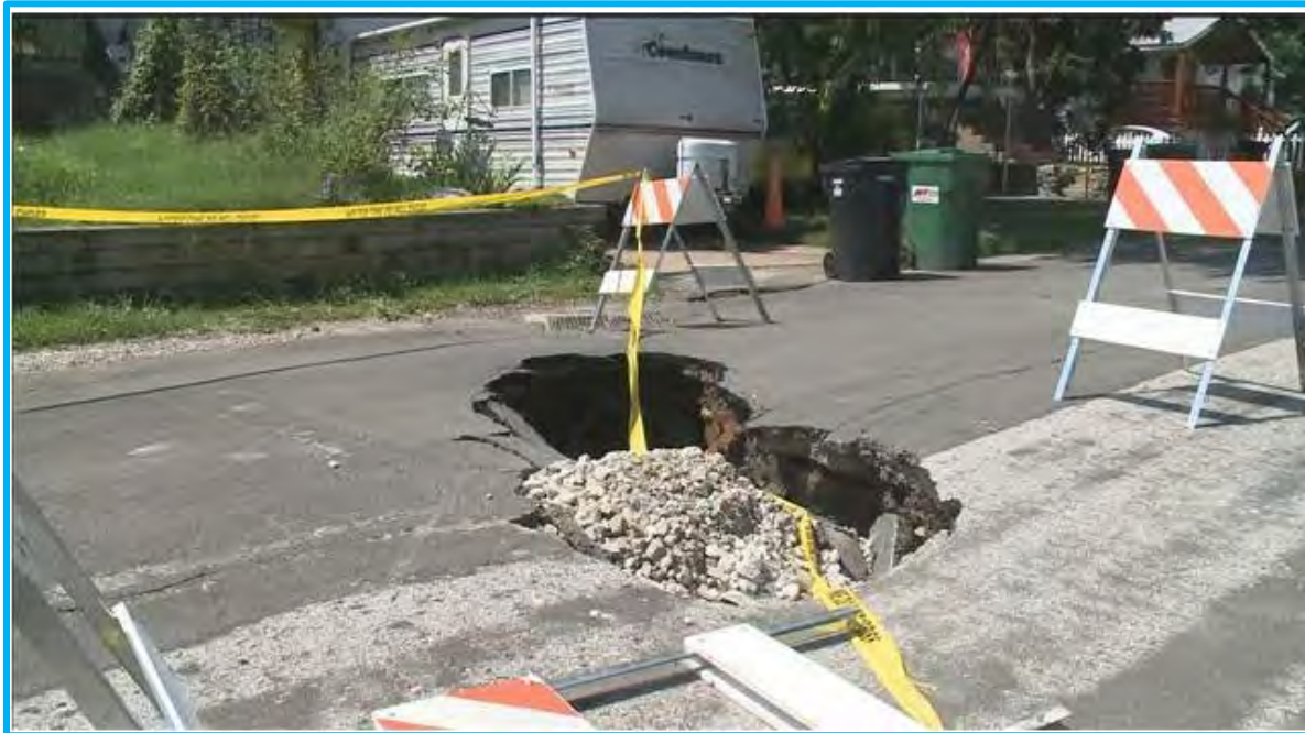
Figure 11. Big sinkhole growing larger in South County, St. Louis County, MO (KSDK).
