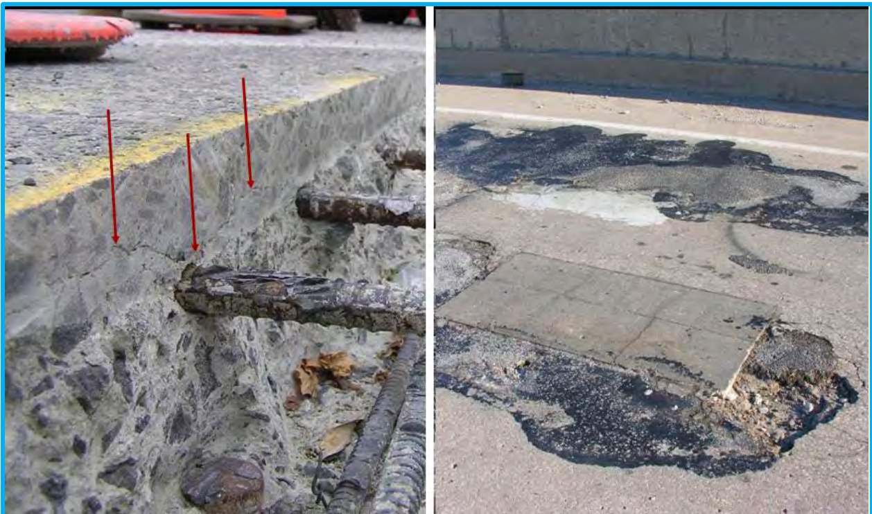
Figure 6. Steel corrosion and delamination (left) and spalling (right). Gucunski N. (2009).
