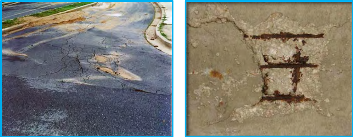
Figure 5. An example of asphalt & concrete deterioration.
