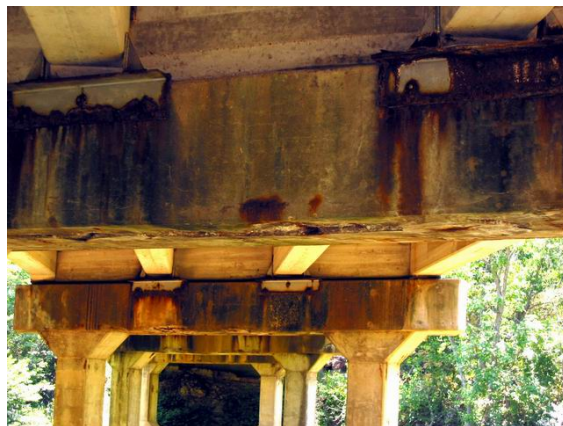
Figure 3. Condition of bents
