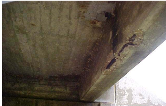
Figure 2. Condition of exterior girder
