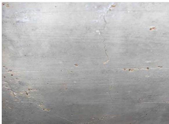
Figure 3. Condition of deck. Longitudinal cracks
