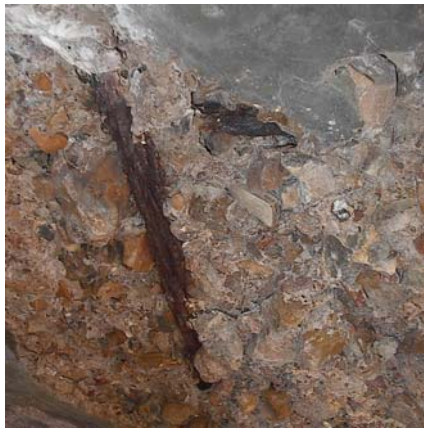
Figure 2. Condition of deck. Corrosion of steel reinforcement
